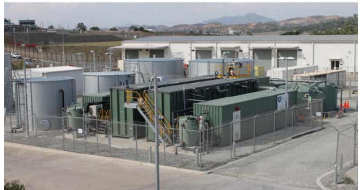
Membrane Bioreactor Sewage Treatment Plant installed on site in Port Moresby
